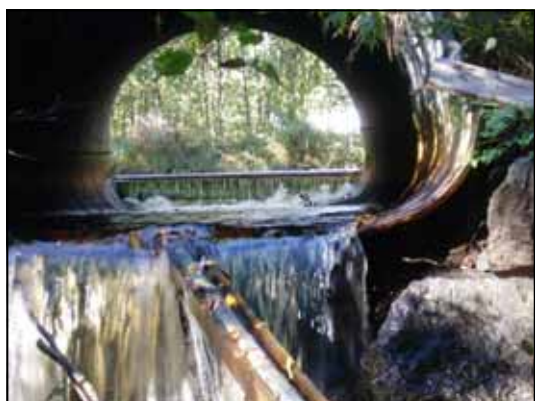
Figur 9. Vandringshinder (tabell 3, hinder 6).
